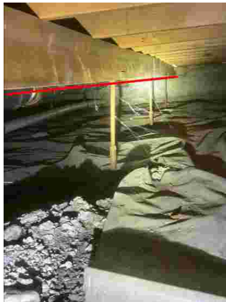
Flooring support uneven
