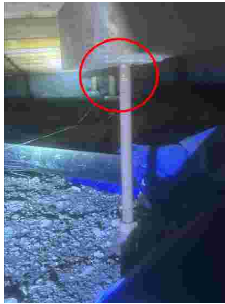
Rust present at threads.
