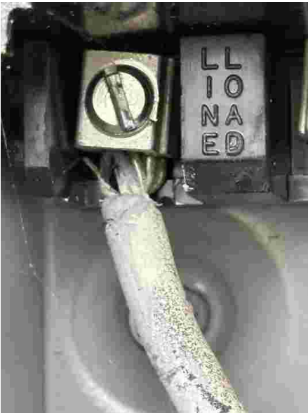
Aluminum wiring to AC unit
