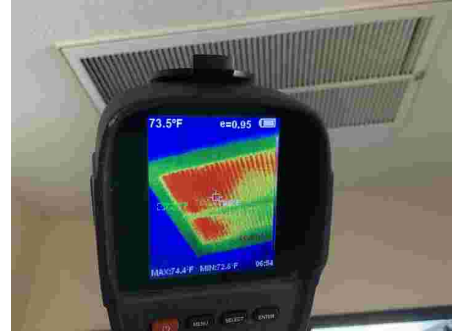
Intake air is 73.5deg
