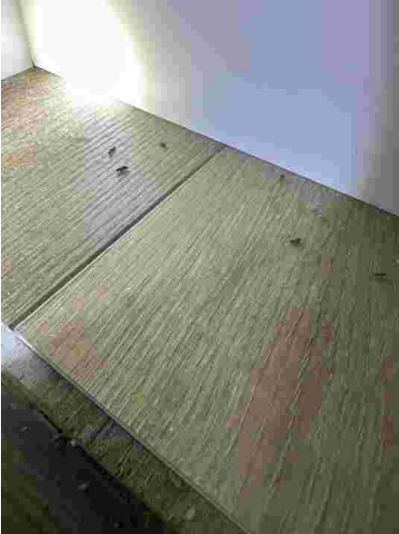
Mice droppings on new floors in front bedroom.
