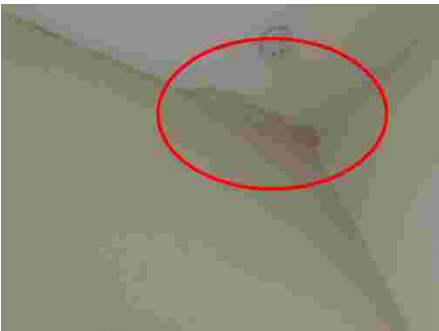
Crack/uneven ceiling in master bedroom.
